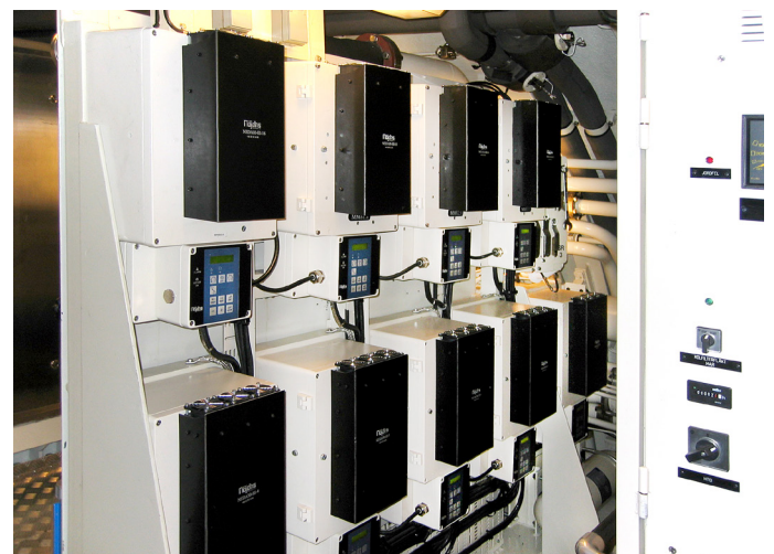
DC-AC-converters installed in a submarine.
